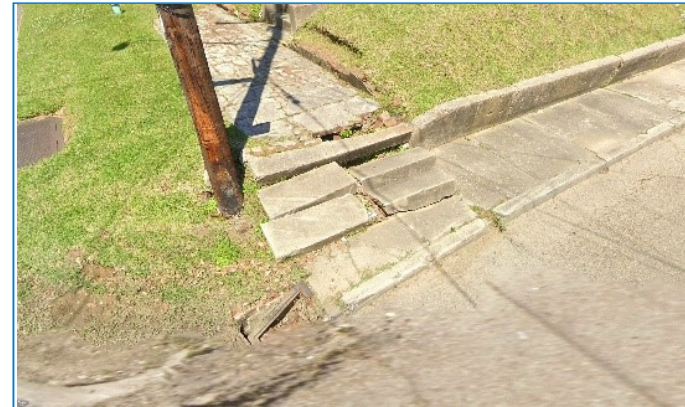
Existing non-compliant sidewalk
